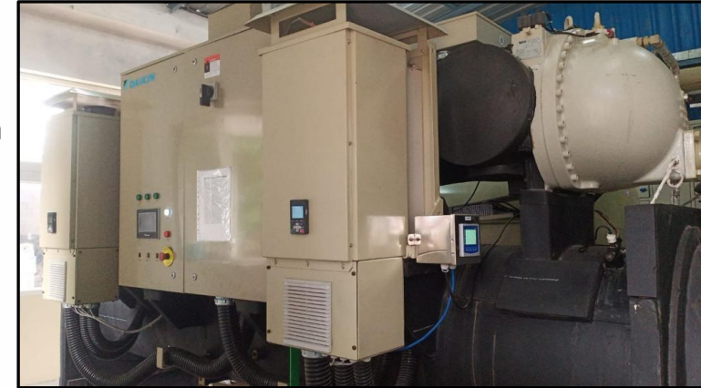
350 TR WATER COOLED SCREW CHILLER
