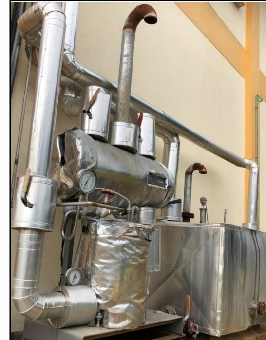
CONDENSATE RECOVERY PUMPS (PPPPU)
